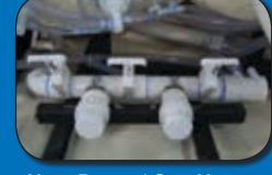
Heat Pump / Gas Heater Connections
